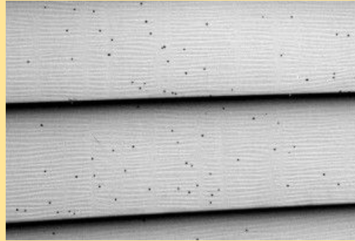
Fungus on siding:
